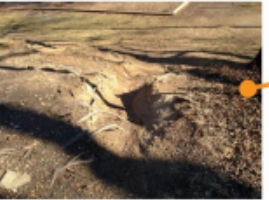
Erosion at cut-thru
